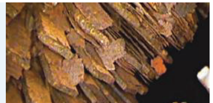
Before. Impacted deposits on finned tubes.
